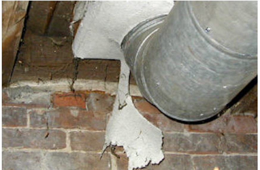
Suspect asbestos containing material (damaged) observed around heat duct in basement.
