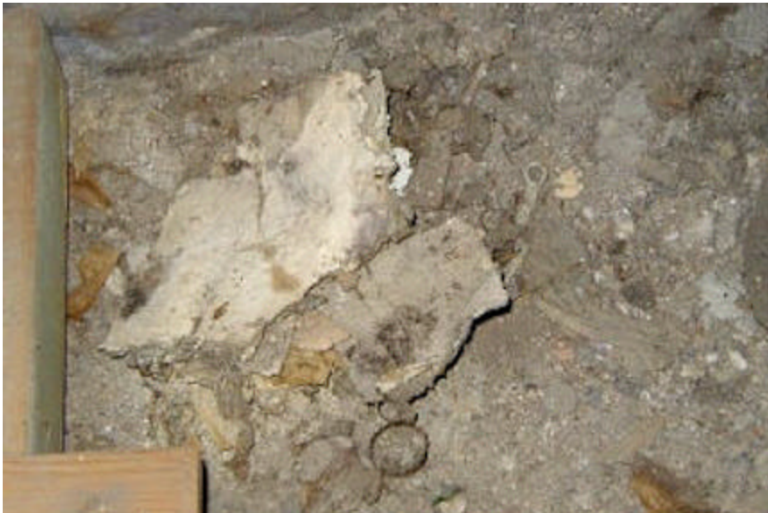
Suspect asbestos containing material (damaged) observed in the dirt basement floor.
